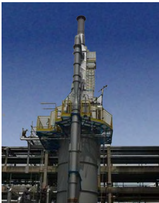
Newly installed super heater
